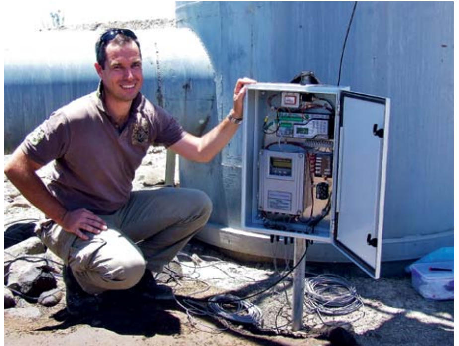
NCEA researchers Gary Sandell and Phil Szabo (pictured) are trialling a pump performance monitor they have developed, to provide data which will be used to examine pump efficiency.
